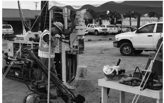
Donny Smith, Assistant Manager, Hydrex Field Services, operating a Geoprobe crawler-mounted rig that was used to demonstrate hollow-stem auger drilling, direct-push technology, and monitor well installation
